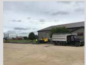
Asphalt work is happening around campus this summer, including Championship Drive and the Shelby Middle School parking lot.
