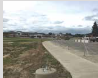
Sidewalks, lighting, and a wider culvert are added to Championship Drive from Shelby Middle School to the new stadium for improved safety.
